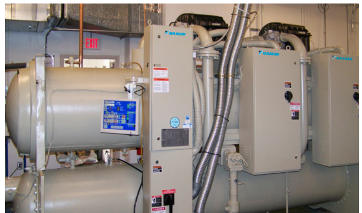
A 387-ton Daikin Magnitude magnetic bearing chiller replaced a 23 year old, water cooled centrifugal chiller resulting in annual energy savings of approximately $79,000.
